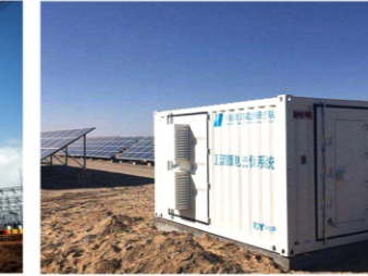
Photovoltaic energy storage system
