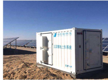
Photovoltaic energy storage system
