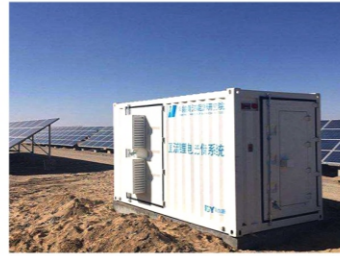
Photovoltaic energy storage system
