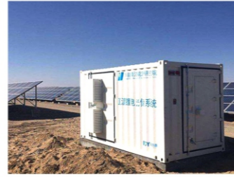
Photovoltaic energy storage system
