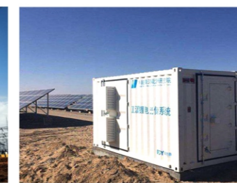
Photovoltaic energy storage system
