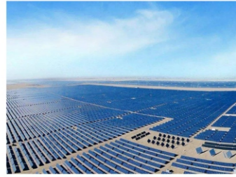
Photovoltaic power station
