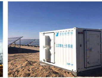
Photovoltaic energy storage system
